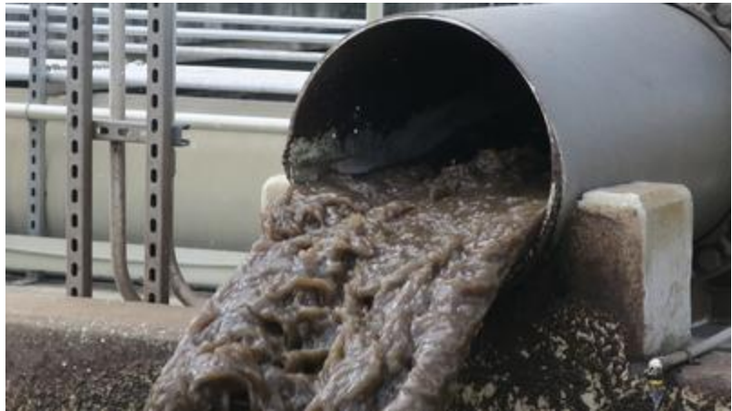
Altamonte Springs was a pioneer in advanced treatment of sewage, converting it to irrigation water.
