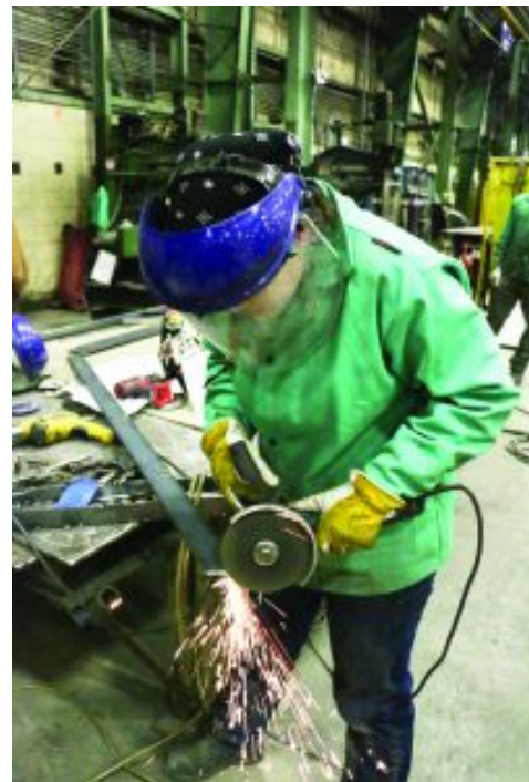
Heather Craig grinds steel at John McDougall Company, a metal fabricator and longtime union contractor.
