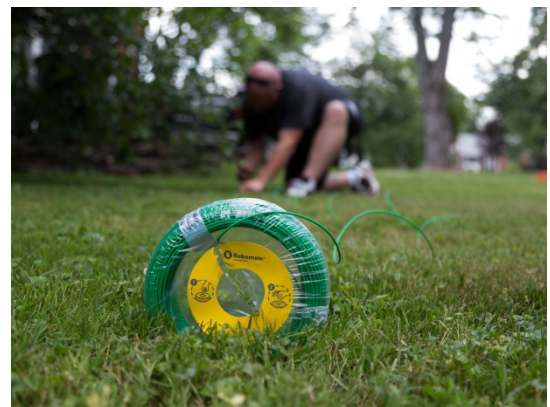
Technical editor Steve Conaway installs the perimeter wire around my front yard. Chris Monroe/CNET
